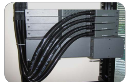
A multi-enclosure Interface kit, breaking out the tubes of an incoming loose tube cable, into 4 enclosures
