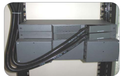
Two multi-cable Interface kits, breaking out 8 incoming loose tube cables into 2 enclosures
