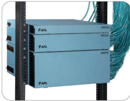
ASCEND Fiber Housings in Rack
