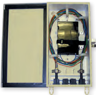
LL-500 with LL-2450 splice tray installed
