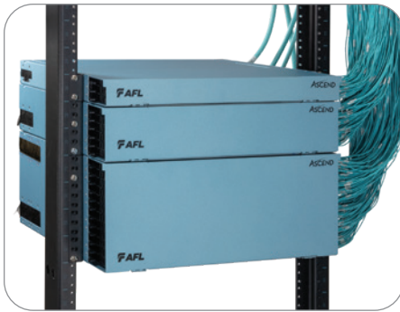
ASCEND Fiber Housings in Rack
