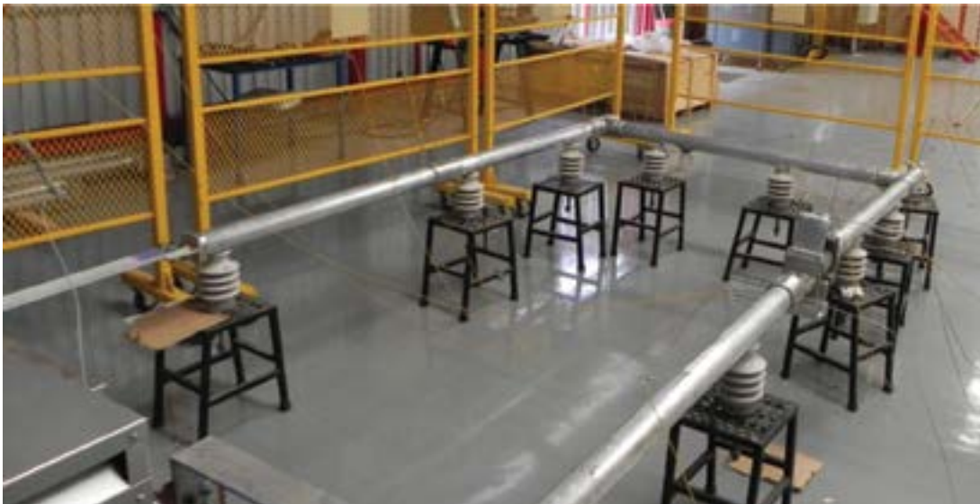
Test loop installed and connected.
