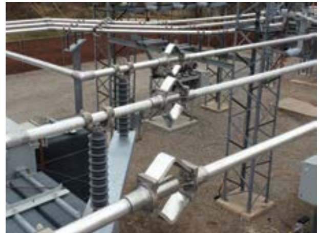
Swage Bus Expansion Terminals installed on a substation at Logan City Light and Power in Utah.
