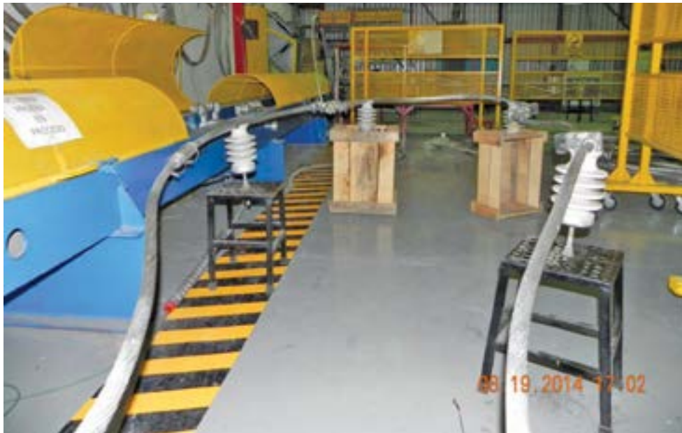
Test loop installed and connected.
