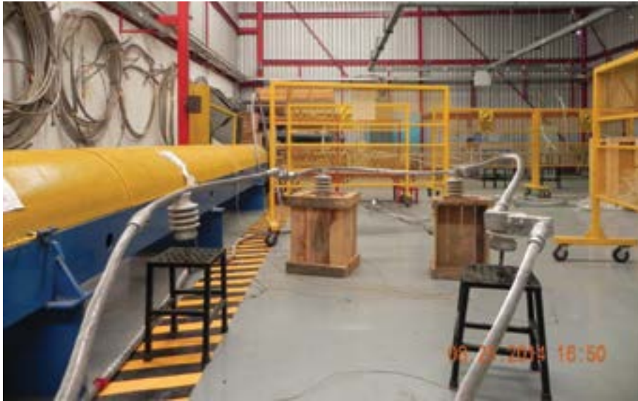
Test loop installed and connected.
